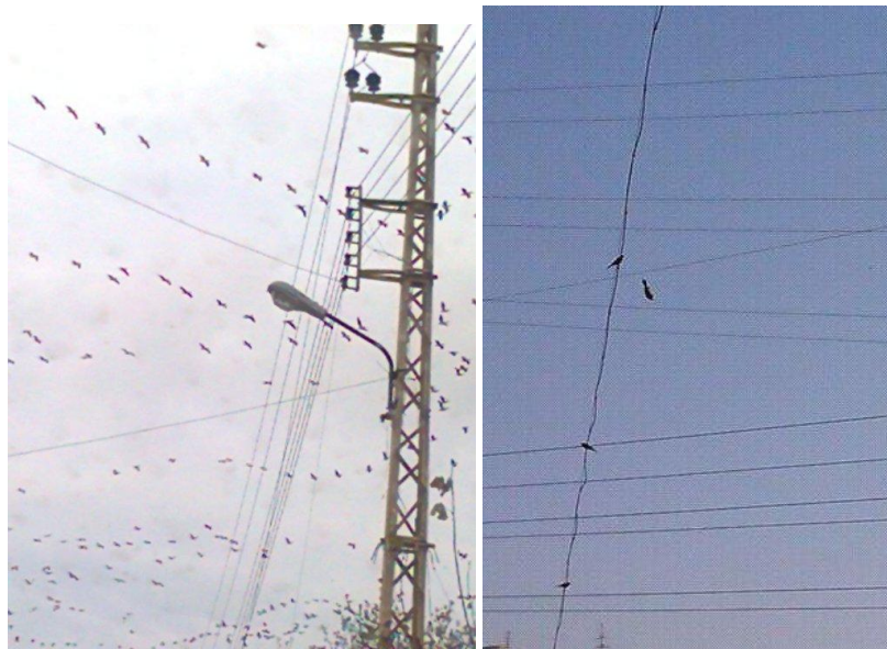
Birds resting on high voltage lines
